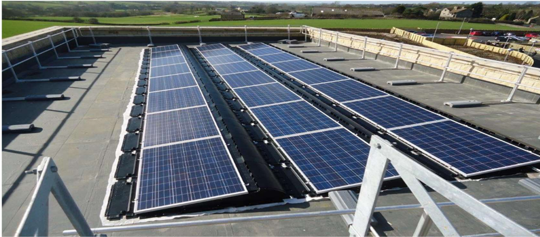
Bentham School – Indicating Photovoltaic Panels to Hall Roof.
